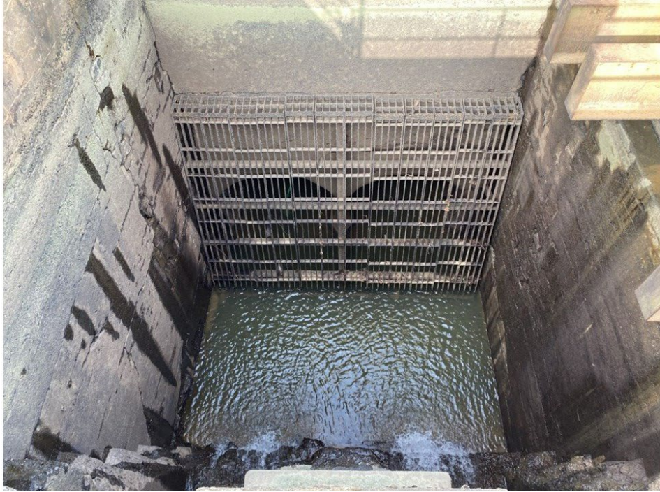
Figure 1.8.3-1. Trashracks located in each of the turbine intake bays at Schoolfield Project.
