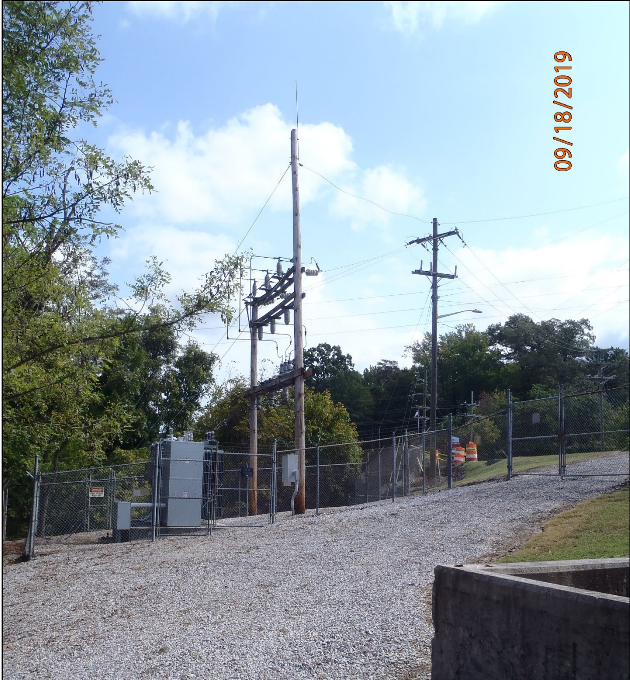
Figure 1.8.7-1. Photograph of the Project's substation.
